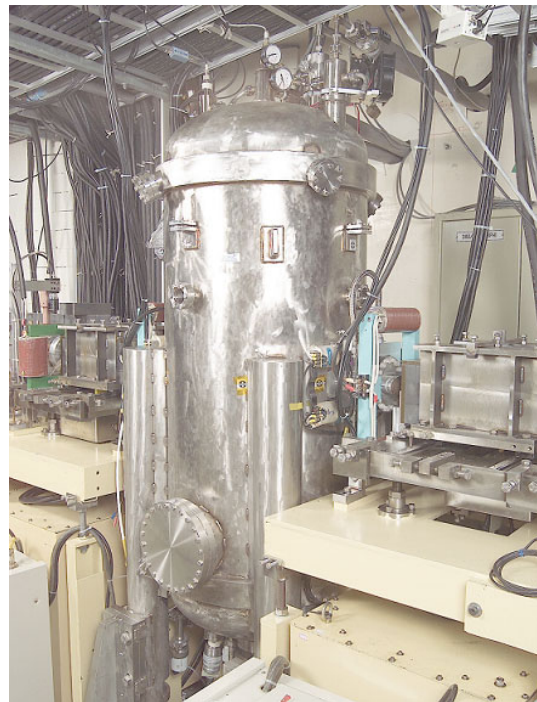
Fig. 3: SWLS was installed in the injection section between kicker 3 and 4. A pair of multipole shimming magnets is mounted on the magnet flange. The cold head of the cryocooler was mounted on the bottom of the magnet.
